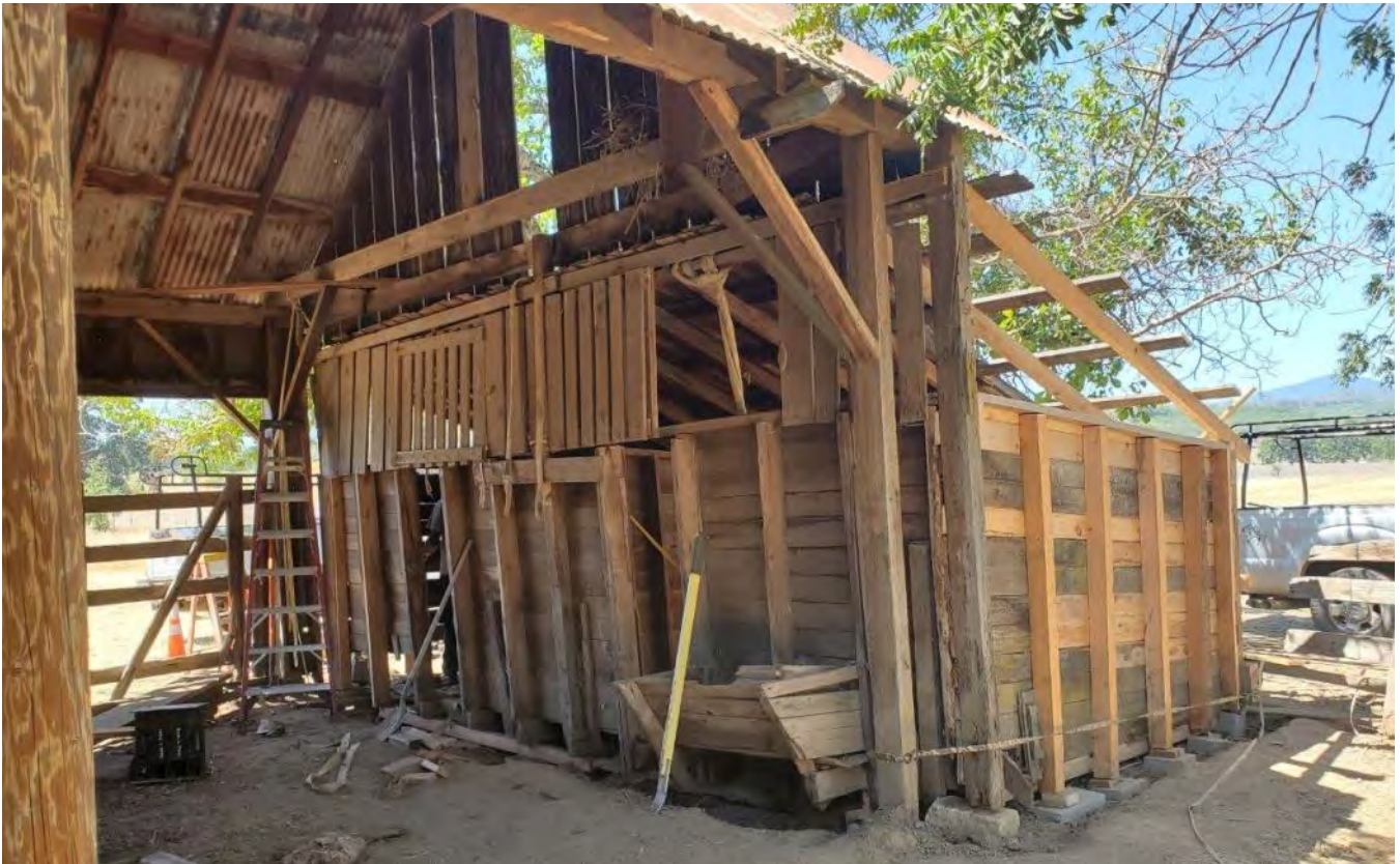
South barn shed shown undergoing repairs. The barn shed is the only part of the building that survived the great snowstorm of 1947.
