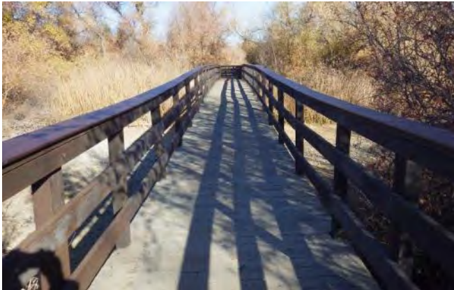
New Trex railings and other repairs made to the boardwalk on Cache Creek Nature Trail.
