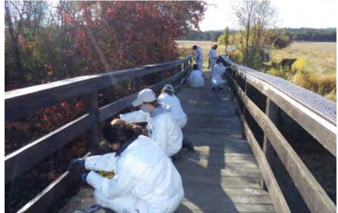
The repairs were made by AmeriCorps volunteers, supervised by State Parks staff.
